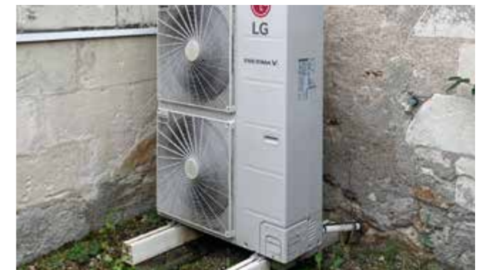
Example of a heat pump installation
